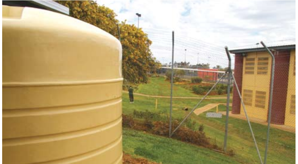
> Large rainwater tanks installed at Junee Correctional Centre form part of the centre's environmental management plan.
